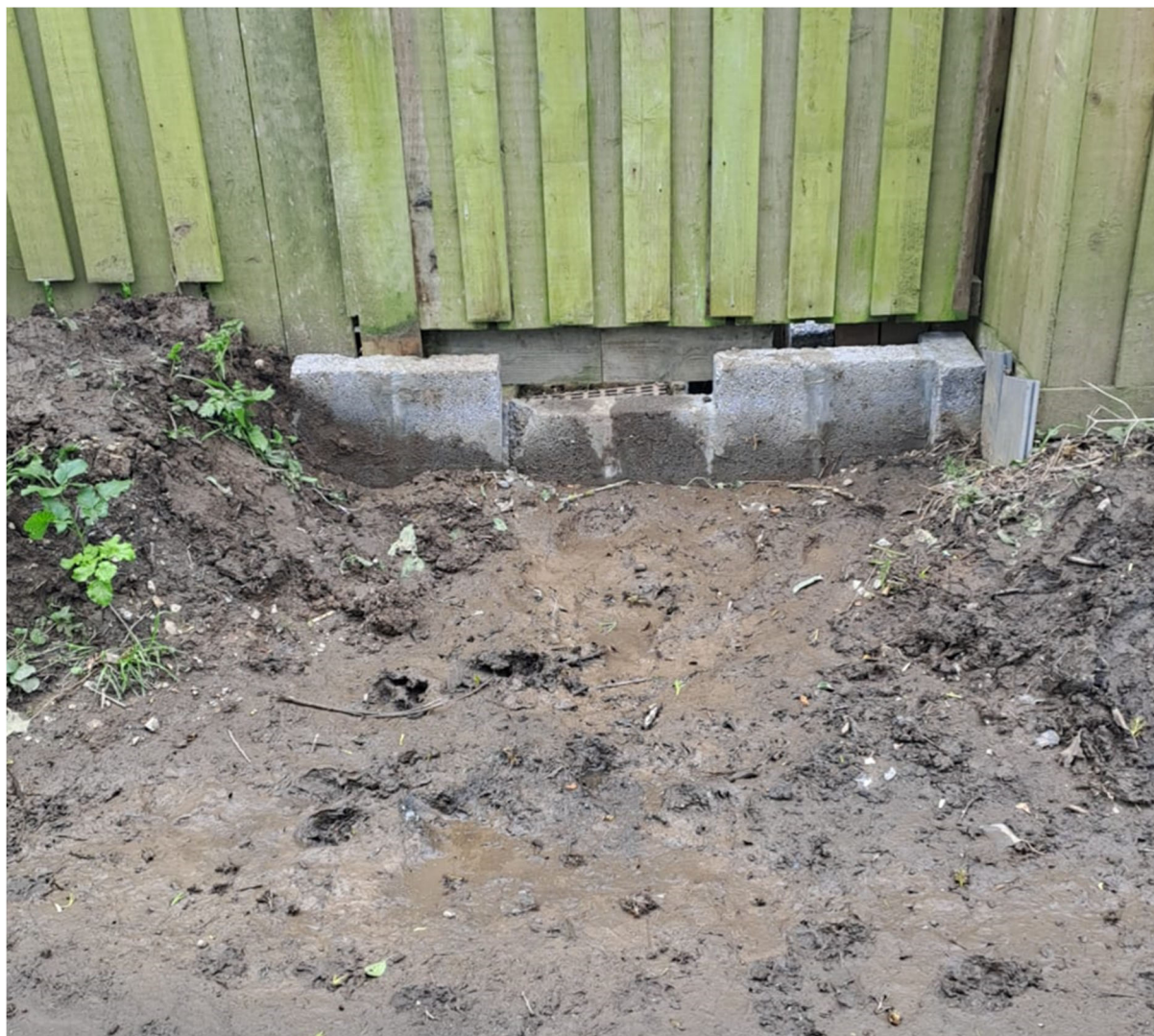
Fig 3. Domestic soakaway installed within the rear garden of 39 Tinney Drive (not accessible behind fence)
